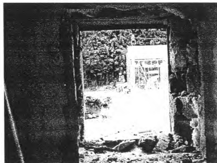
The removal of the boiler opens up a new view of the greenhouse
